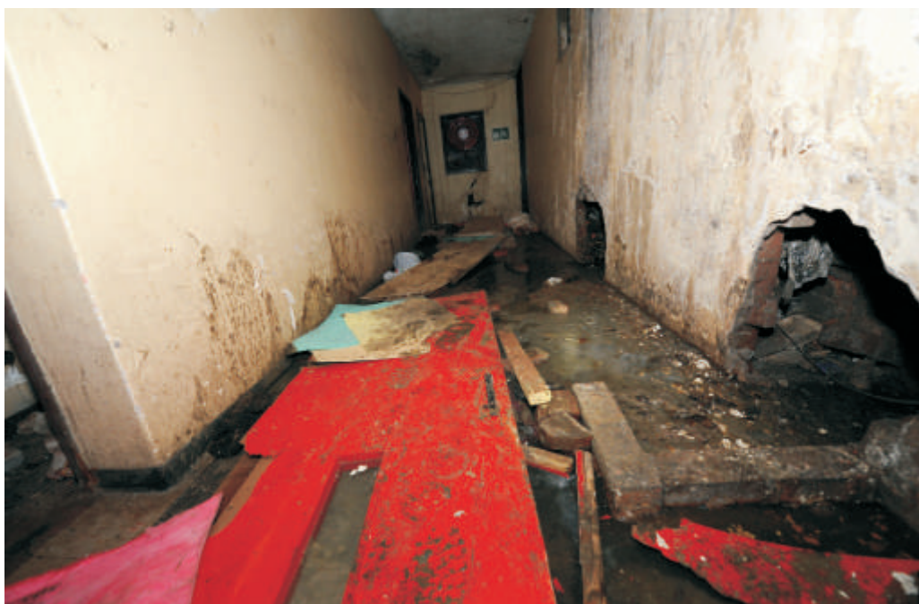
The building is in an awful condition with broken doors and piles of dirt filling the basement.
