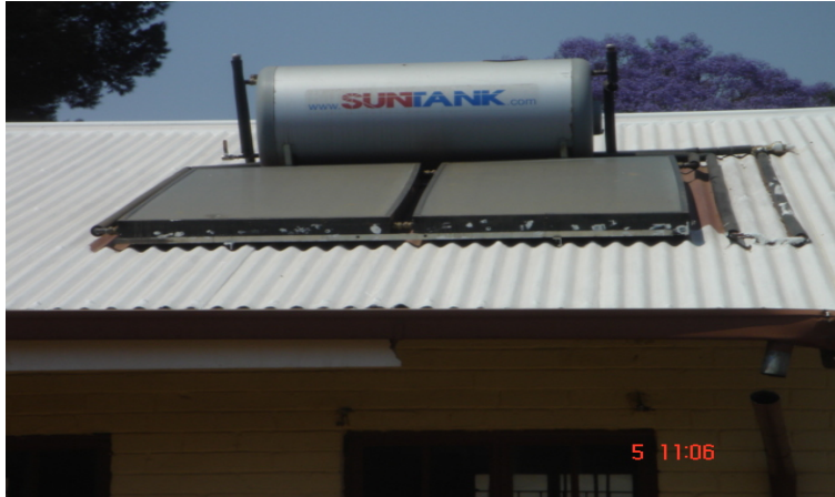
An installed solar water-heating system
